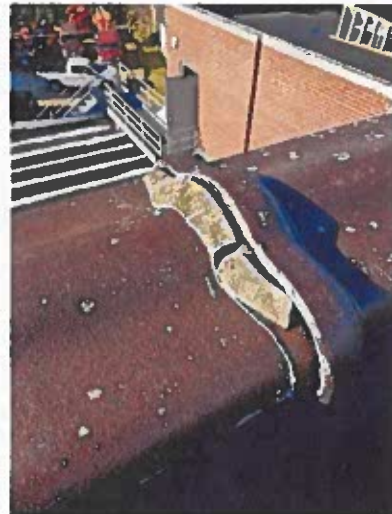
Front upper roof, damaged seal on parapet cap
