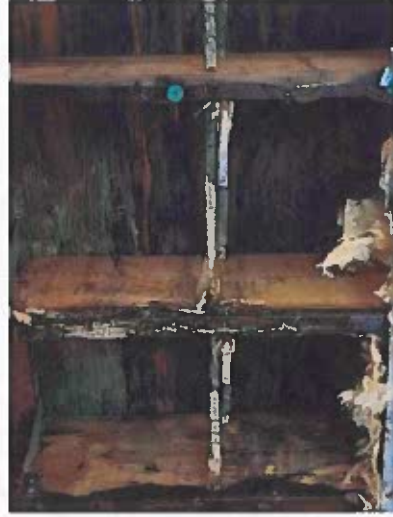
Excessive water damage to decking and rafters
