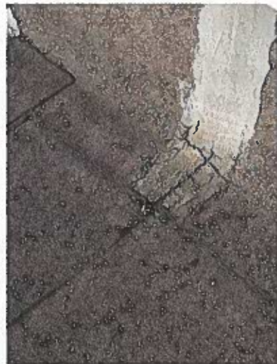
excessive cracking at seam over police station
