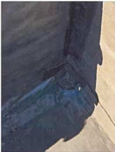
Corner of parapet wall base, front upper roof. Seams starting to separate
