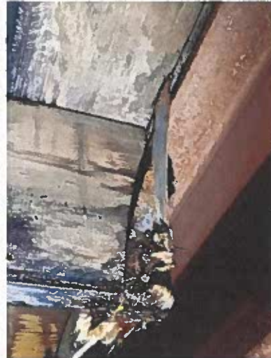
End of rafters show both water damage to the end of the rafter and minor compression. There is excessive corrosion on the joist hanger.
