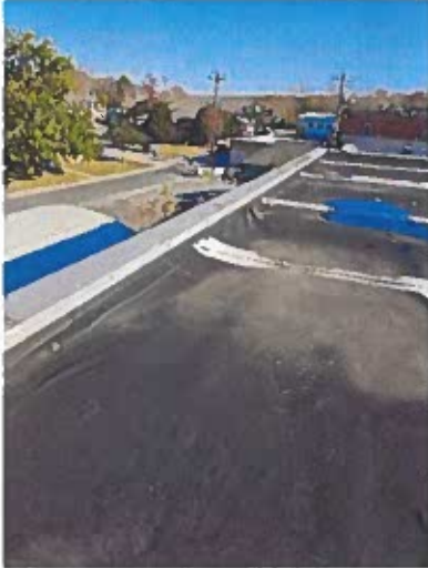
Wrinkles on the rear middle roof. The roofing is pulling away from the side parapet
