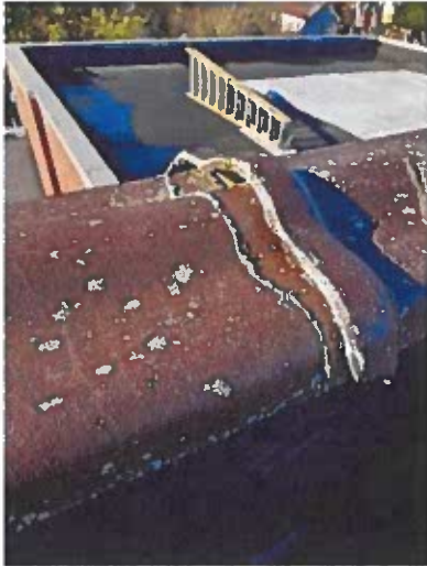
Parapet cap on front upper roof. Missing cement seal around connection point
