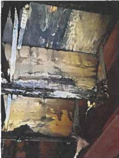
Closer photo of the water damage and biological growth.
