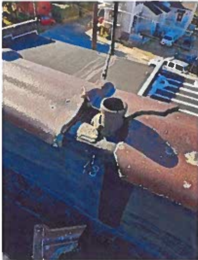
Front upper Roof, damaged parapet cap
