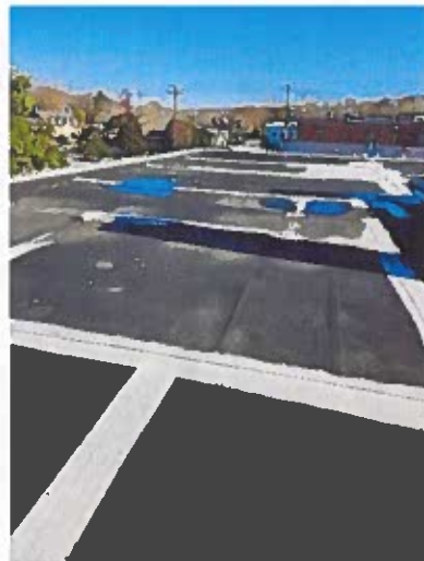
Rear middle roof overview with ponding
