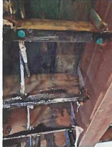
Area of roof structure under leaking Rear middle roof. Area of approximately 10'x10'
